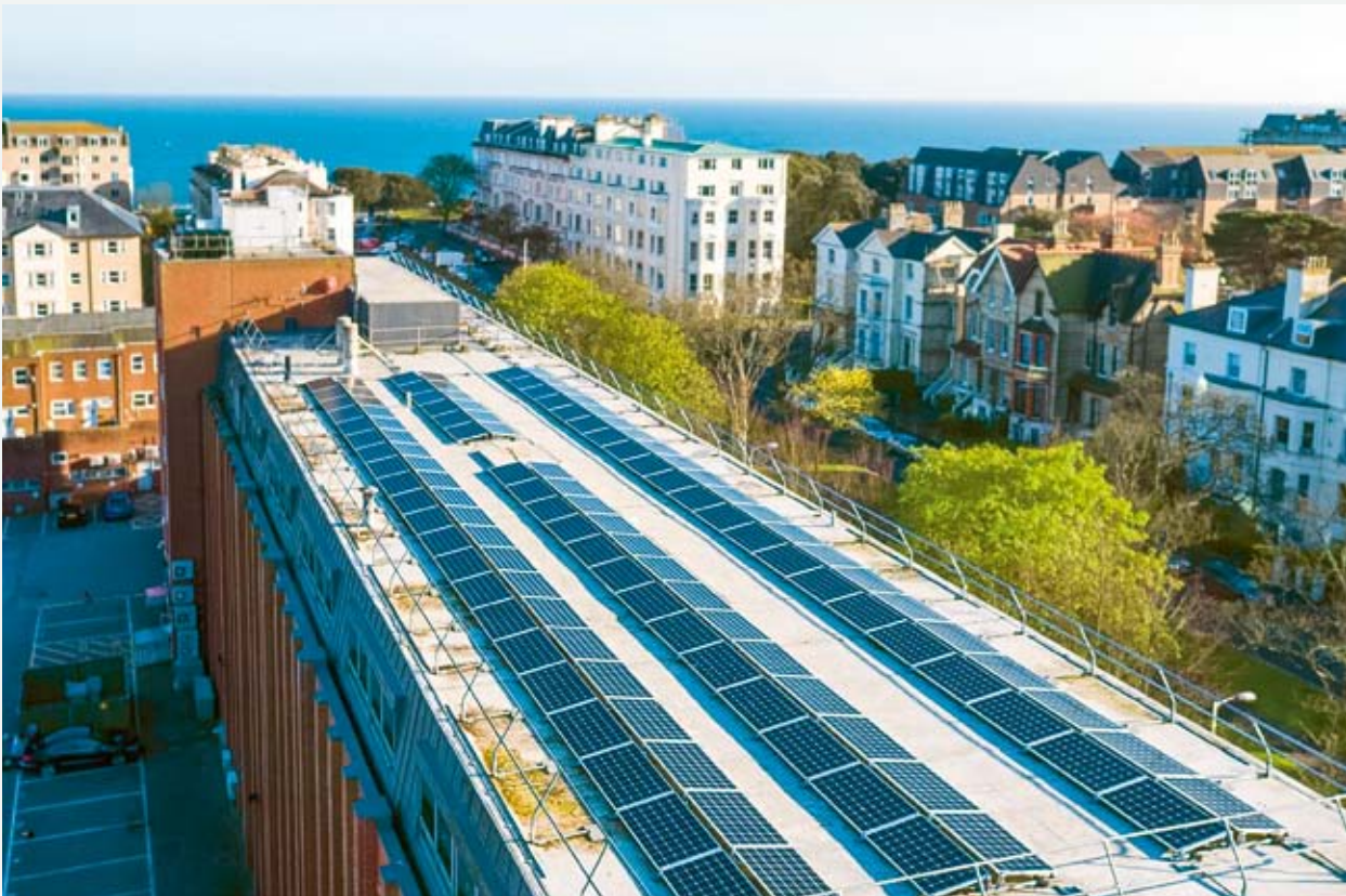
A solar power plant we installed on the roof of our Folkestone office can cover approximately 17% of its power consumption over the year.
