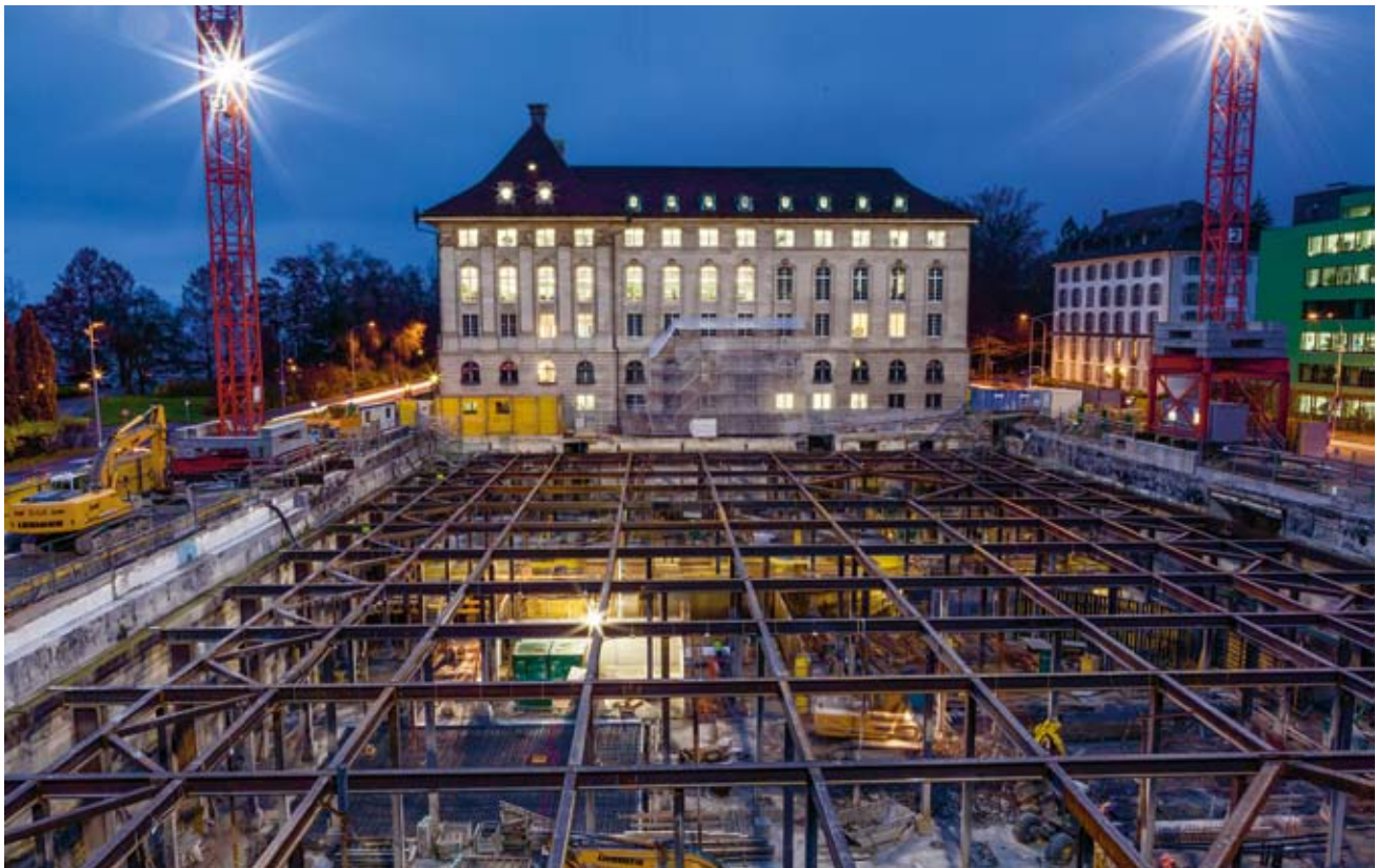
The groundwork is being laid for Swiss Re Next, our new headquarter building that will set a leading example of sustainable construction. The “strut platform” shown in the picture was erected to support and preserve the existing excavation enclosure made of 60 cm thick reinforced concrete. Originally constructed in the 1960s for the previous Neubau building, it is still in superb condition today.
